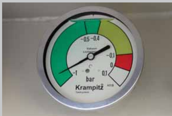
vacuum leak detection, system control
